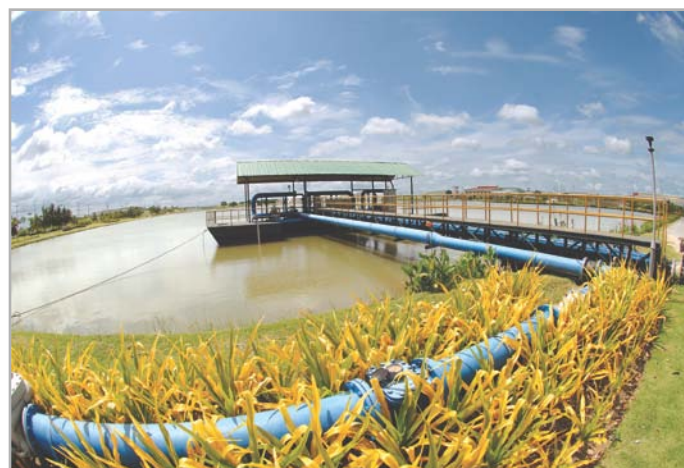
Amata City Treatment Plant, Thailand
